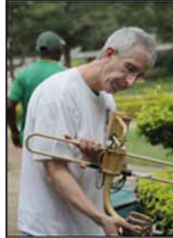
2013 Malawi TV Transmitter Install
